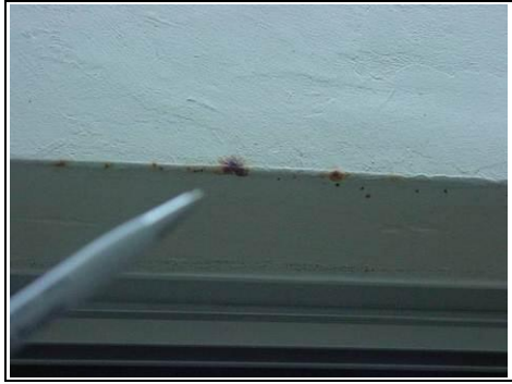
Rusting to corner beads
