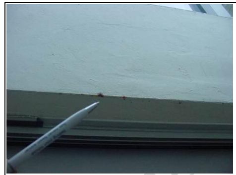
Rusting on the corner bead.
