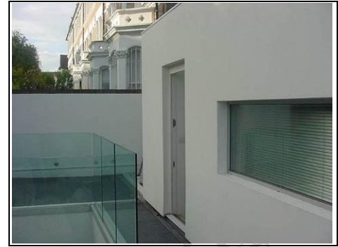
No drip detail above the window
