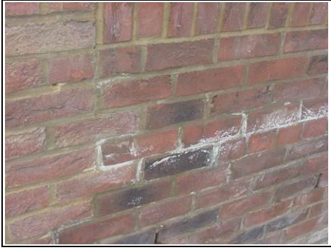
Efflorescence on wall
