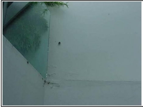
Blistering to rear light well right hand side
