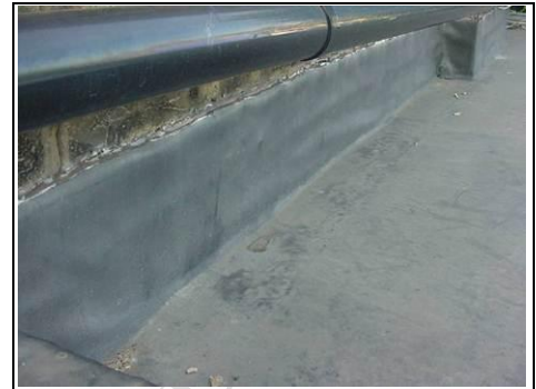
Flashing on the roof where it meets the building next door. We would prefer this to be lead.
