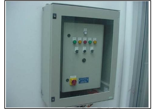
Waste water pump control box
