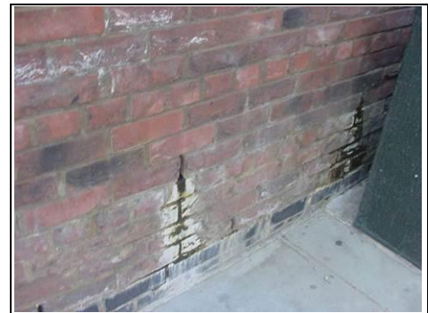
Weep holes that have not been cleaned up
