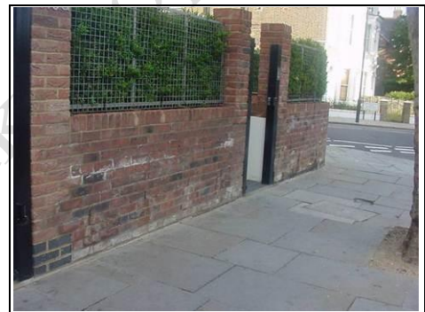
Front wall has problems with water coming out of it
