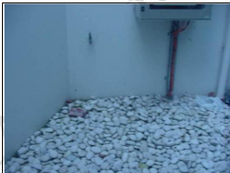
Bottom of the rear light well where we were getting high readings
