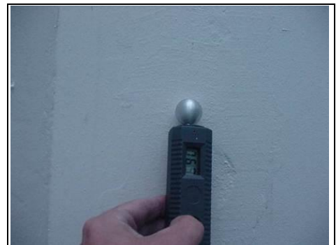
Testing with the damp meter – reading of 69
