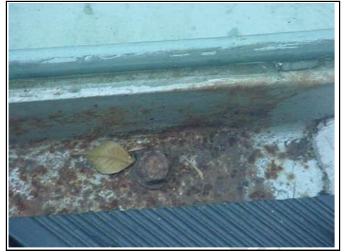
Rust to the base of the rear light well
