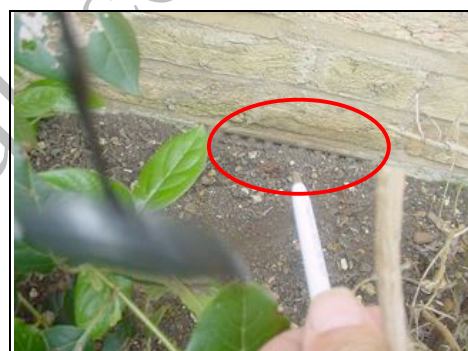
Air brick – ground level needs to be reduced
