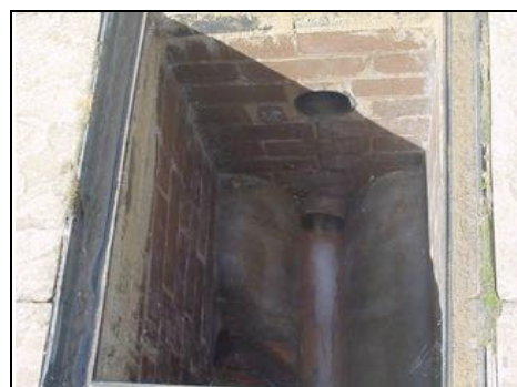
Front left hand manhole
