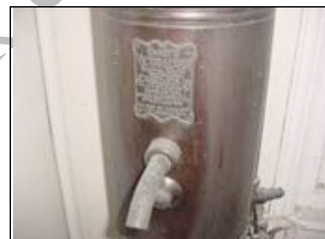
Very old Victorian water heater
