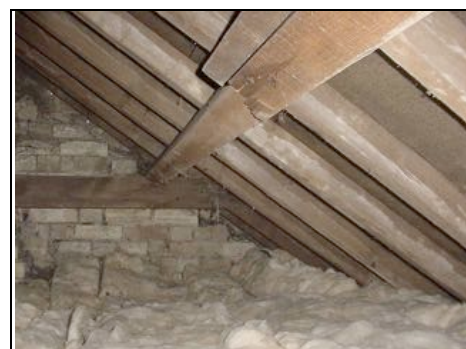
Long length of purlins without support
