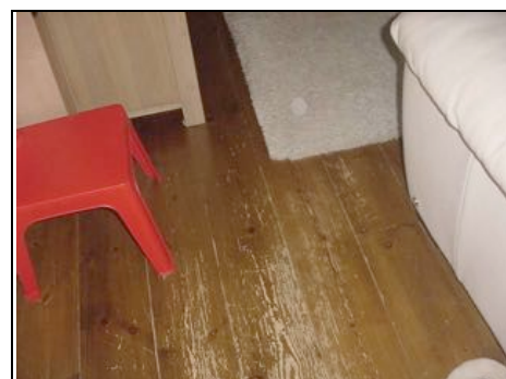
Marks to the floor in the lounge
