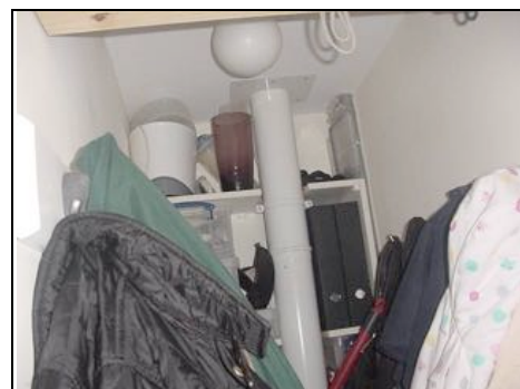
Stored items in boiler cupboard
