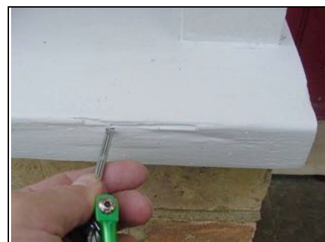
Deterioration to windows
