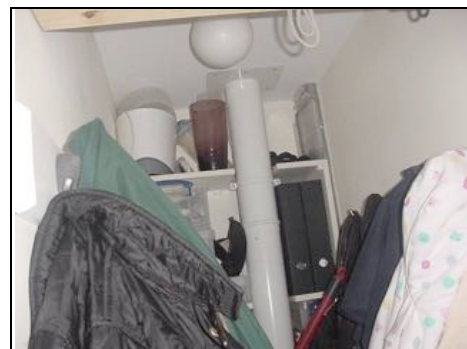
Stored items in boiler cupboard
