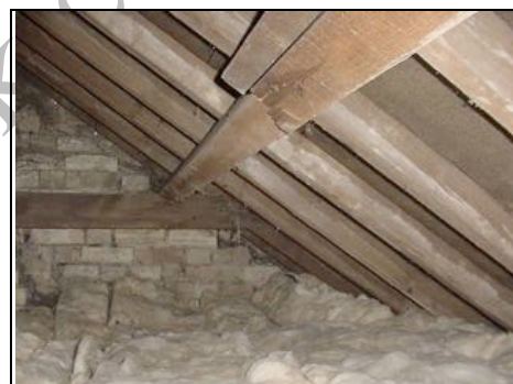
Long purlin without support
