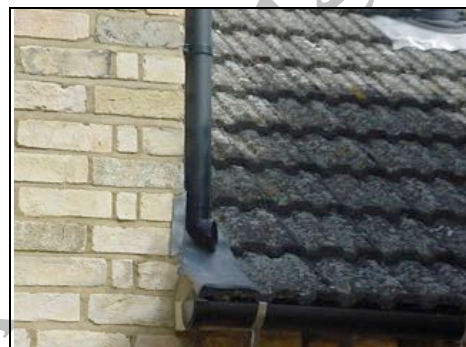
Surcharging gutters and downpipes
