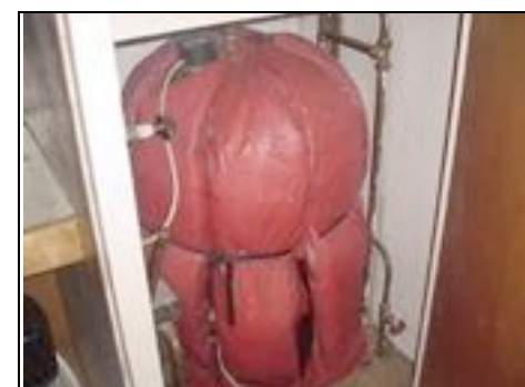
Older style cylinder with loose insulation jacket
