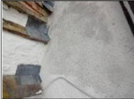
Hairline cracking to right gable ~ Aerial View - 360 Photo ~
