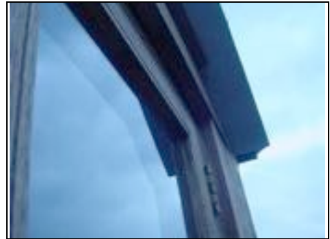
Windows need re-staining
