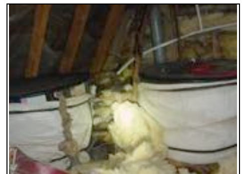
Water tanks in middle roof
