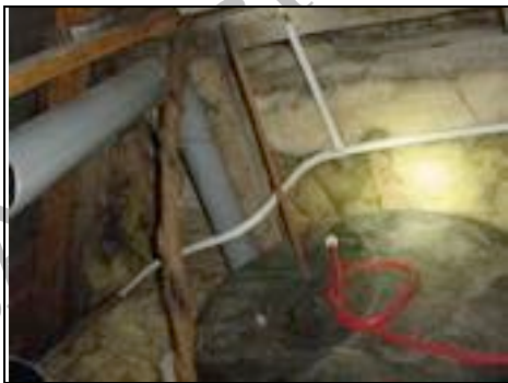
Soil and vent pipe
