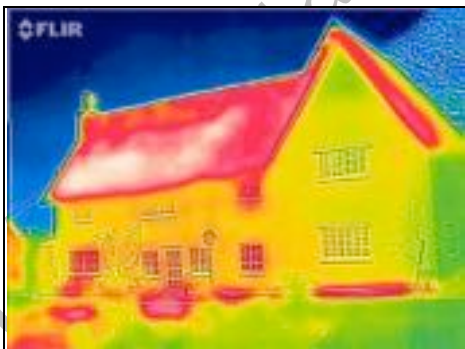
Heat coming out of floor, windows and roof to rear of property and little sign of the timber frame
