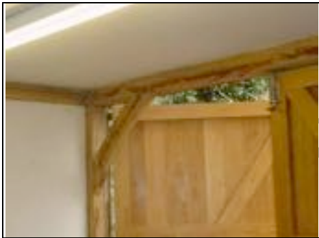
Dampness coming into garage
