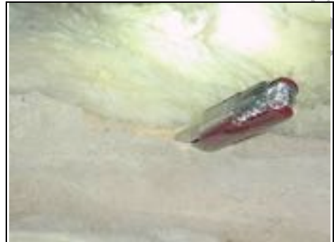
Woodworm/rot in timber in middle roof where it meets left roof
