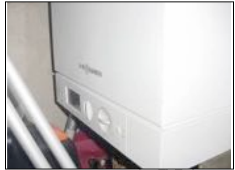
Viemann Boiler in services room
