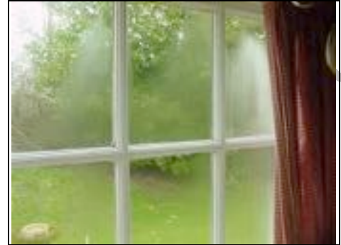
Condensation to windows in kitchen
