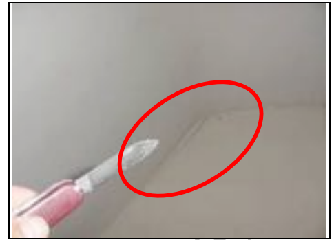
Cracking in far right bedroom
