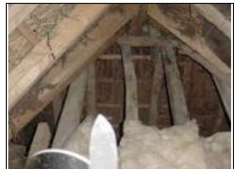
Deterioration/twisting to timbers in left roof
