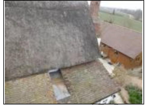
Displaced tiles and in need of repair ~ Aerial View - 360 Photo ~
