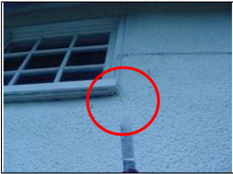
Cracking to the window
