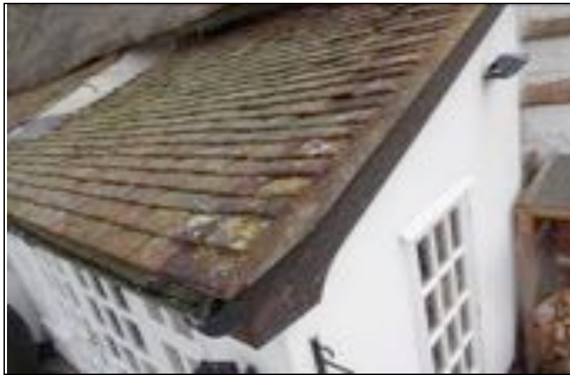
Spalling to tiles ~ Aerial View - 360 Photo ~
