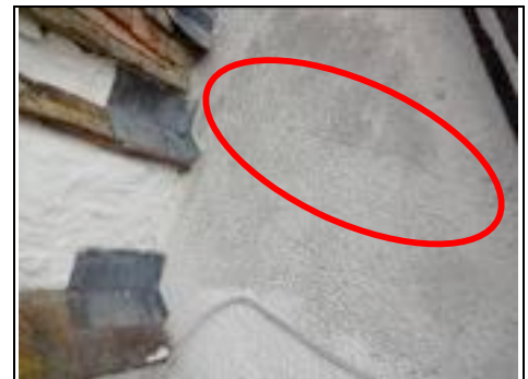
Hairline cracking to right gable ~ Aerial View - 360 Photo ~
