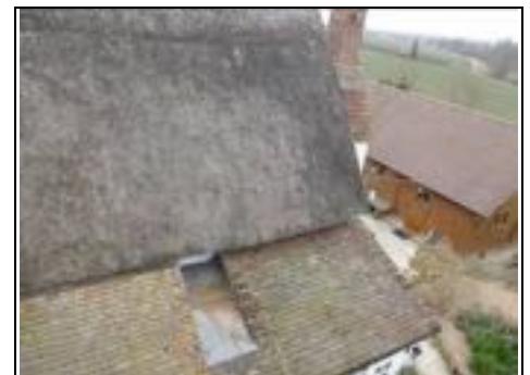
Displaced tiles and in need of repair
