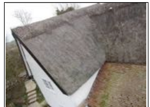
Thatch ridge disintegrating and dampness within thatch ~ Aerial View - 360 Photo ~
