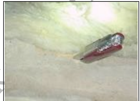
Knife going completely into timber common rafter
