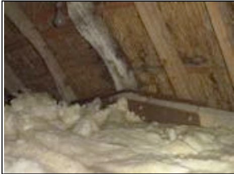
Brace at base of timber in left roof
