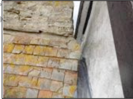
Gap between chimney and main building
