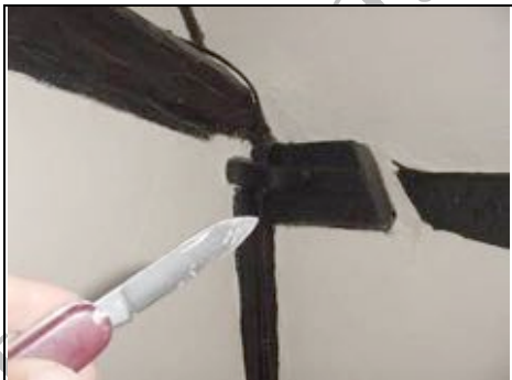
Infill panel with metal brace
