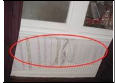
Drying washing on radiators can cause condensation
