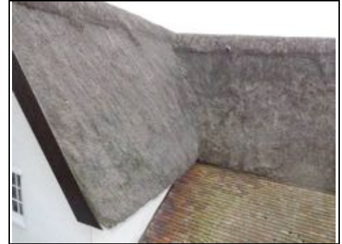
Thatch in poor condition
