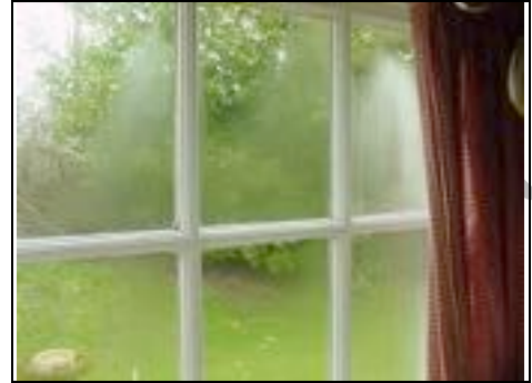
Condensation to windows in kitchen
