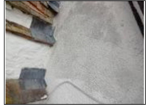
Mastic on lead to right gable
