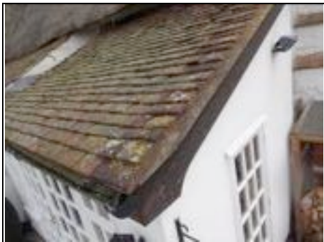
Spalling to tiles ~ Aerial View - 360 Photo ~
