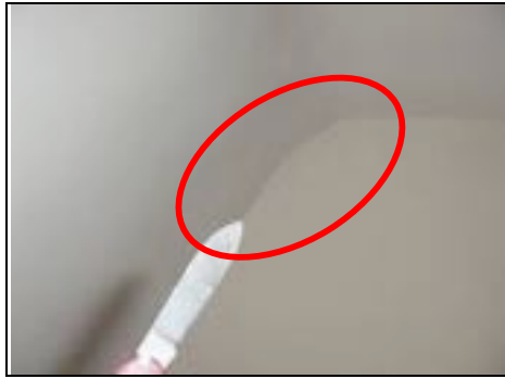
Hairline cracking in master bedroom
