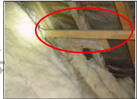
Purlin missing replaced with very thin purlin Plastic sheeting
