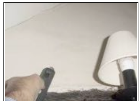
Dampness coming through plaster in right bedroom
