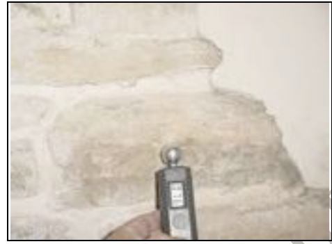
Dampness in stone
