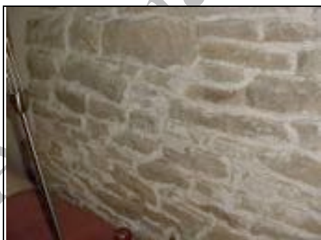
Dampness coming through and various repairs
