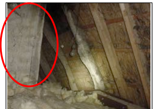
Hidden chimney/smoke hood
