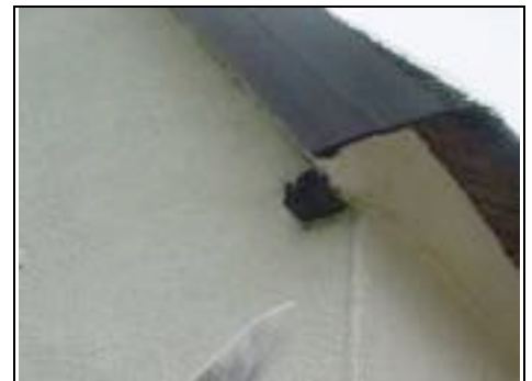
Purlins can be seen protruding out of walls which can lead to rotting
