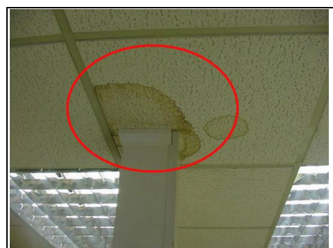
Staining to the ceiling caused by water pipes leaking above the shop ceiling and needs repairing.
