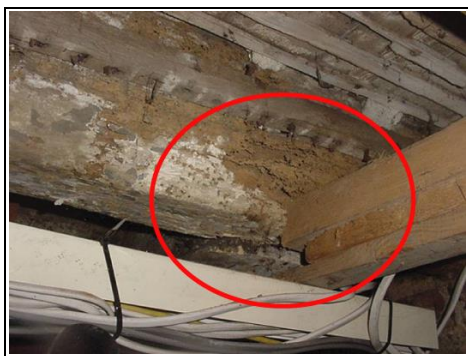
Timber in the basement deteriorating from dampness and woodworm
